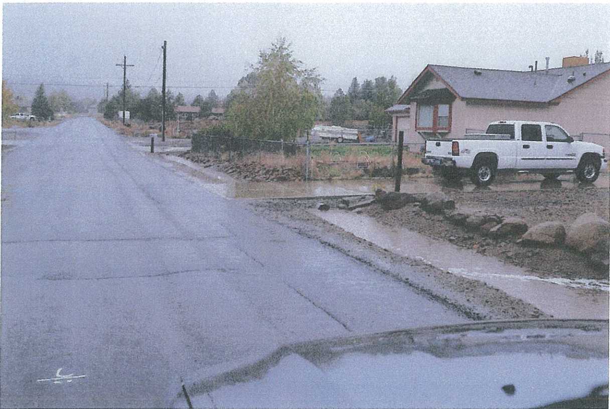
Storm water discharge through a 12" culvert on Shawna Lane. Photograph taken October 16 th 2016 at 2:02 PM.
