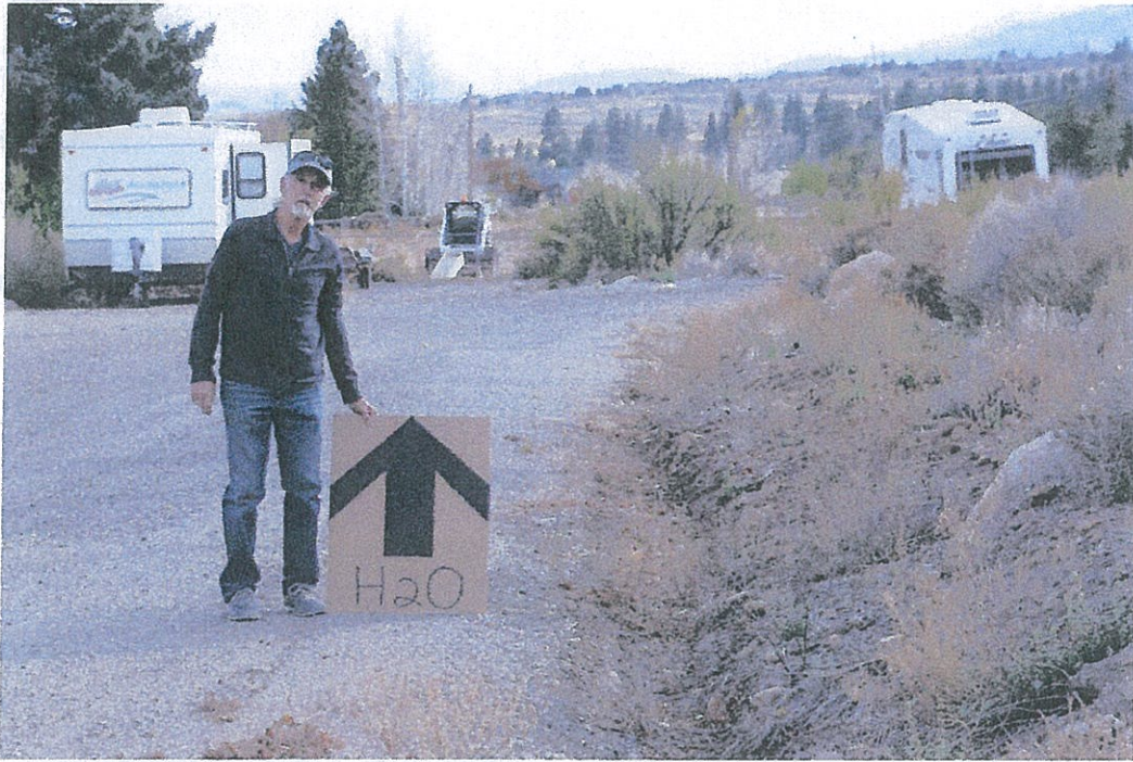
P5. Overflow path 1 in poorly defined ditch on private property.
