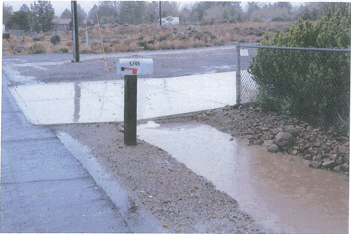
Photograph taken on October 16 th , 2016 at 5:26 PM of 12" culvert on Shawana Lane. Note that discharge is at capacity for this storm water system.
